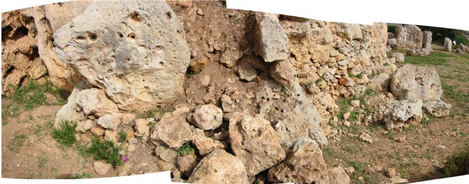
73. View of 2003 collapse in south-west elevation – composite
