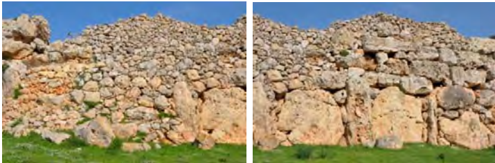
10. South-west elevation – previous collapse
