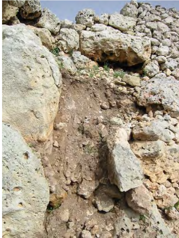
74. Detail of 2003 collapse
