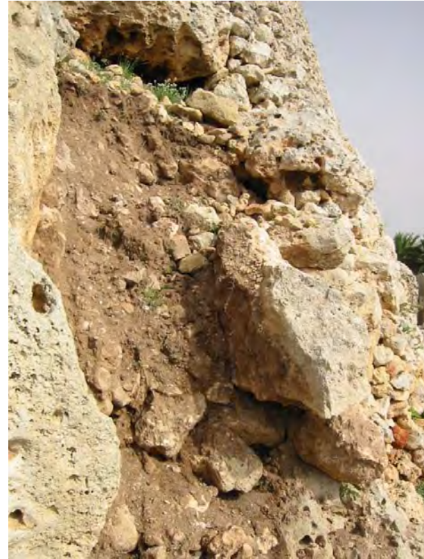
75. Detail of 2003 collapse
