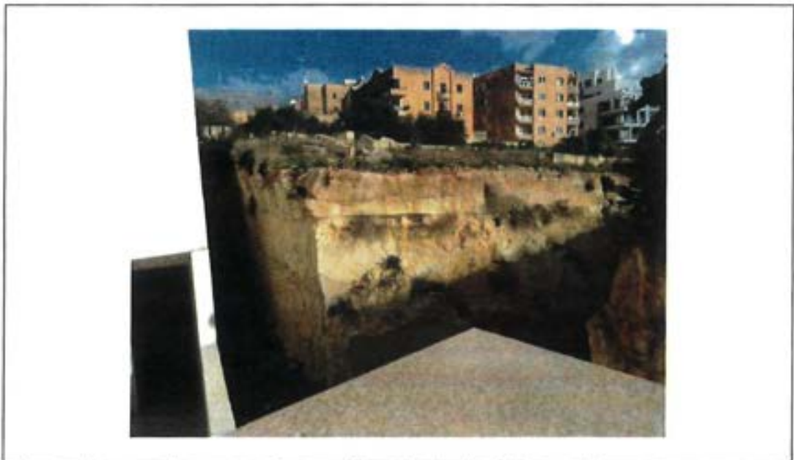
Photo 8: third party rock excavation along rear of site on the Triq Charles Sciberras side.
