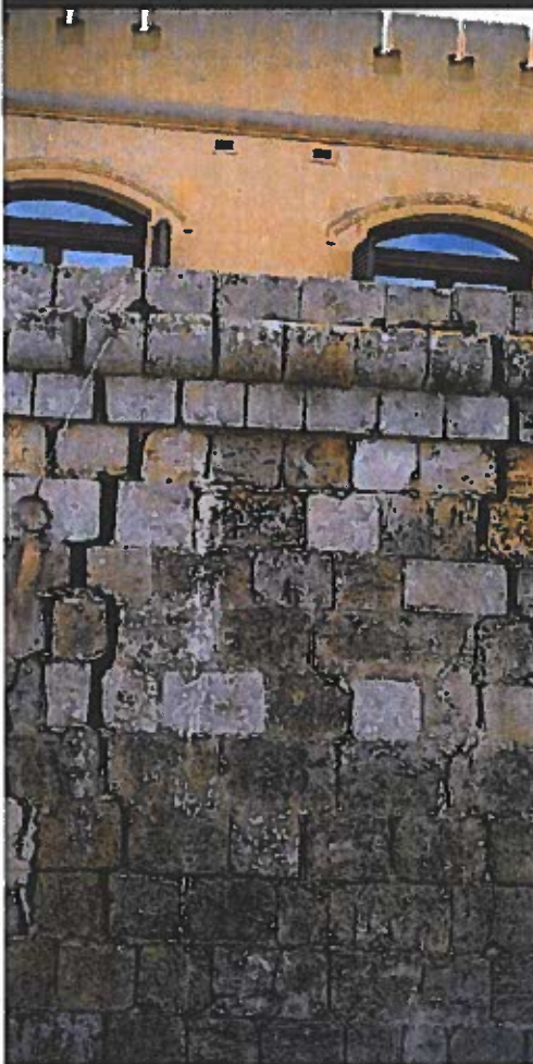
The Fort Chambray project developers have defended restoration works despite worrying cracks around the historic fort. Photo: Matthew Mirabelli » See story on page 5
