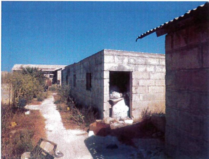
Photo 12: North & west elevation of structure No 18, as indicated in table 1, and its outside area
