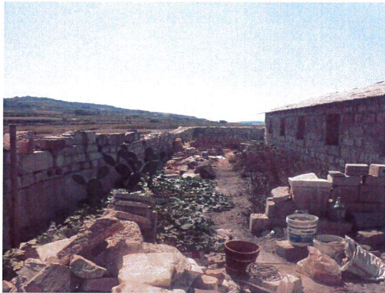
Photo 9: South elevation of structure No 14, as indicated in table 1, and its outside area next to the boundary wall
