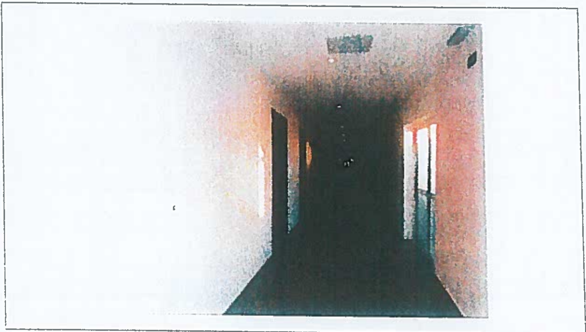
Photo 4: note existing state of slightly upgraded hotel corridor with abutting doors to rear guest rooms.
