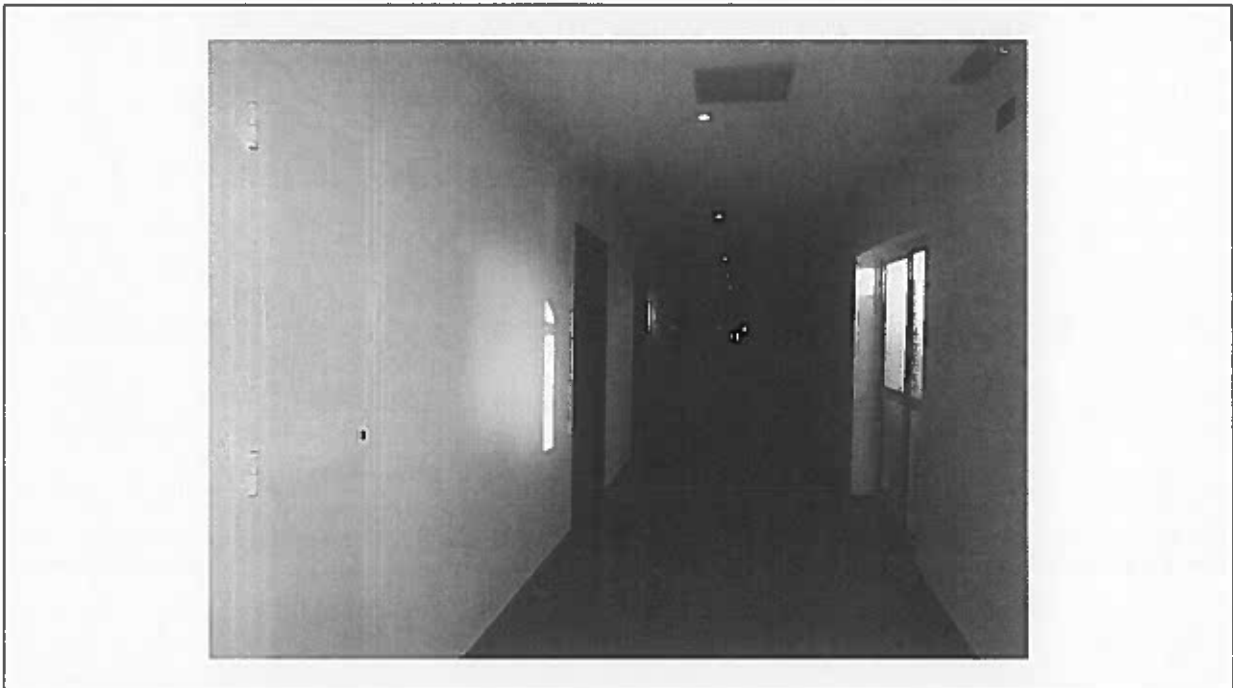
Photo 4: note existing state of slightly upgraded hotel corridor with abutting doors to rear guest rooms.
