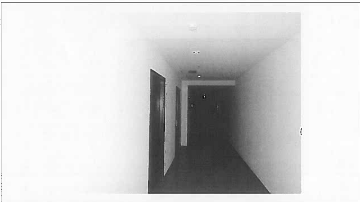
Photo 8: note existing state of hotel corridor with abutting doors to rear guest rooms.
