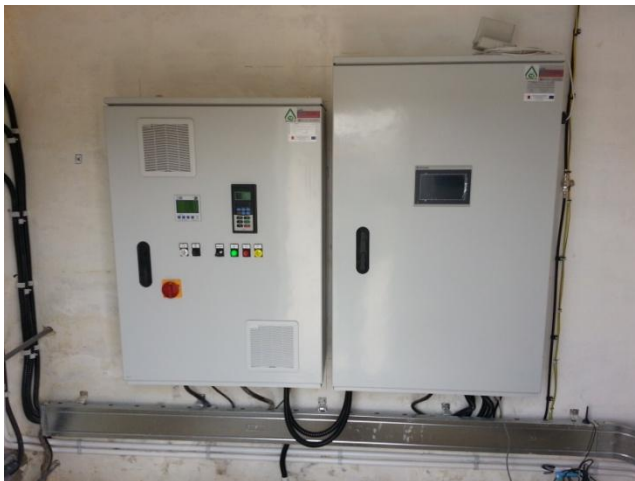
Tat-Torba Borehole Electrical Installation (VSD + Telemetry O/S)
